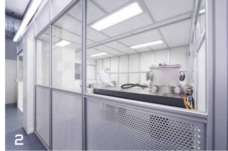
2 ISO5 cleanroom as a room-in-room system in the thermal/vacuum laboratory.
